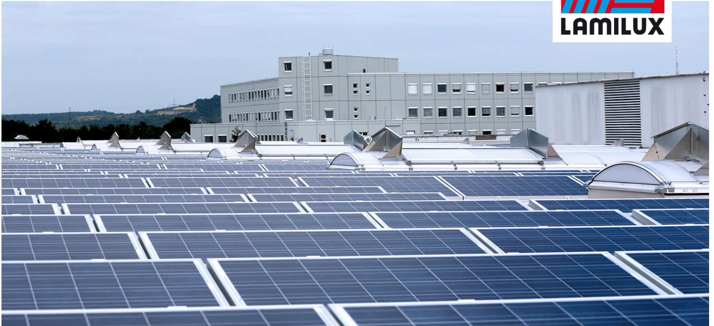
Schneider Electric, Regensburg, Germany
