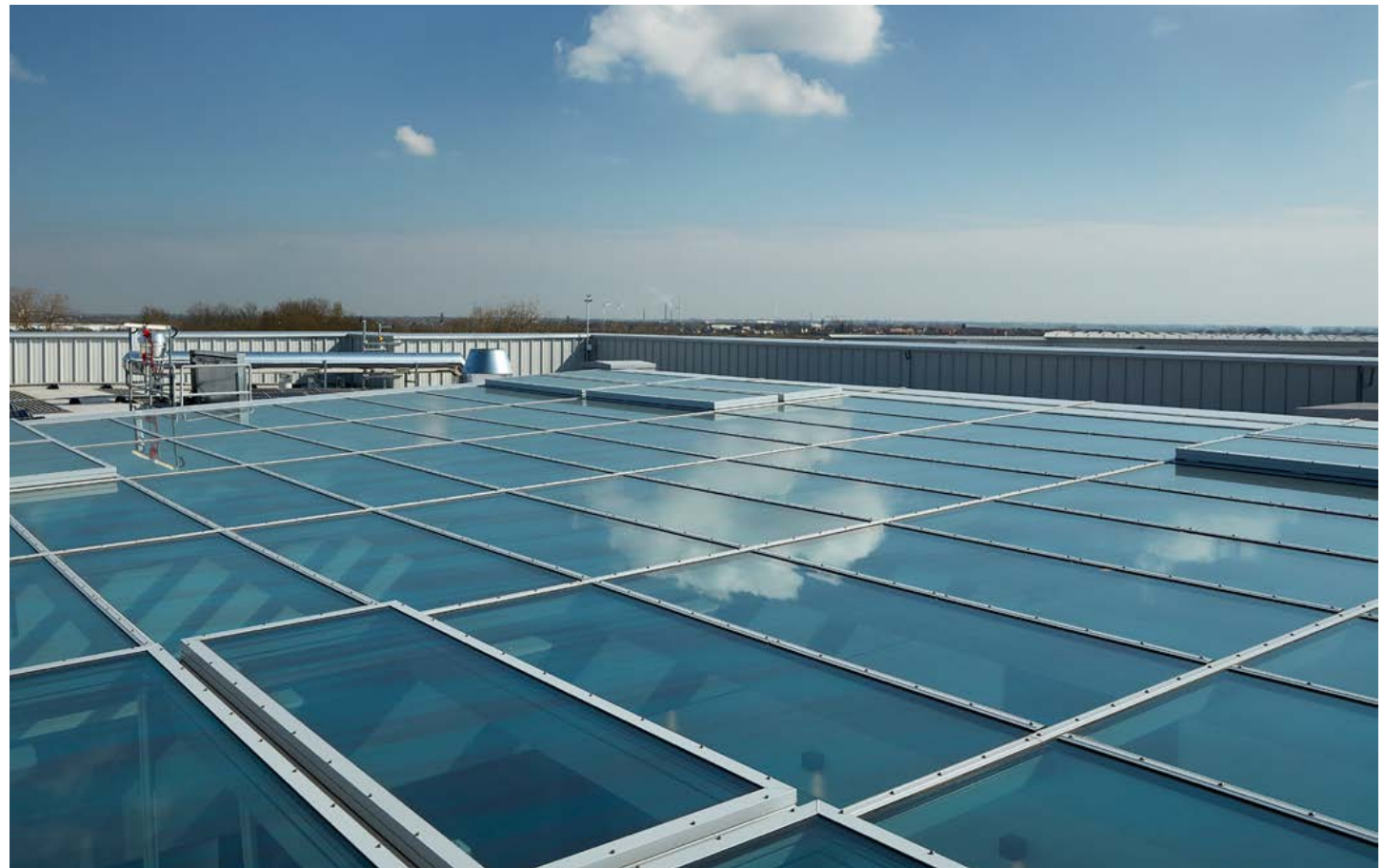
LAMILUX Glass Roof PR60 on the flat roof of "British Sugar"
